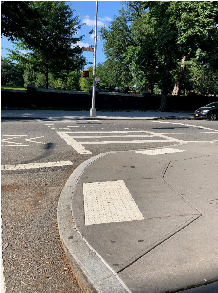
Figure 99 Detectable warning unit at a sidewalk intersection.
