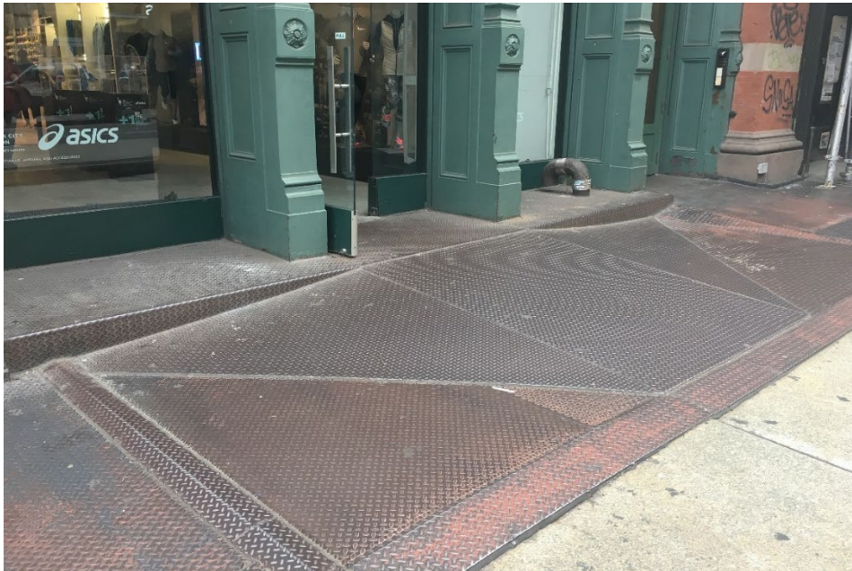
Figure 3. Ramp without handrails
