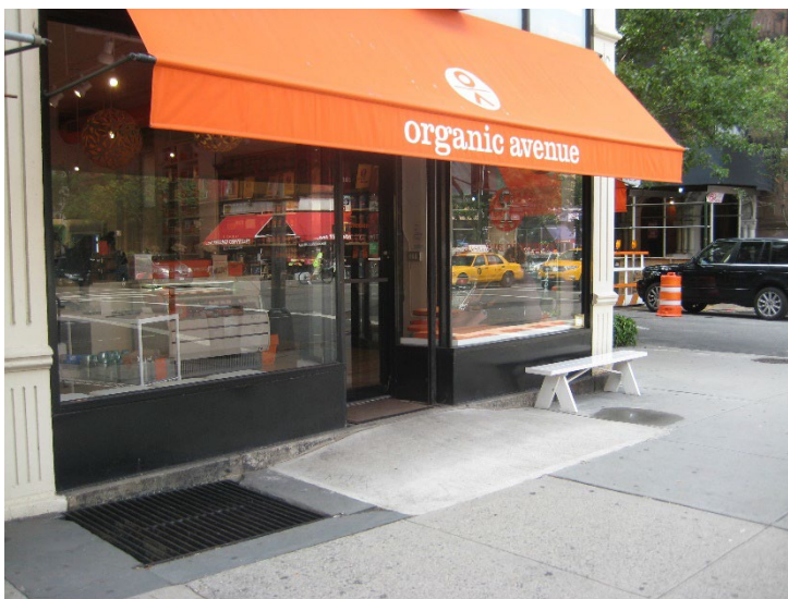
Figure 10. Concrete sidewalk sloping away from a storefront entrance.
