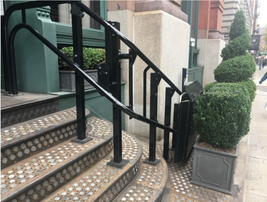
Figure 5. Mechanical lift finished to match the surrounding materials and recede from view
